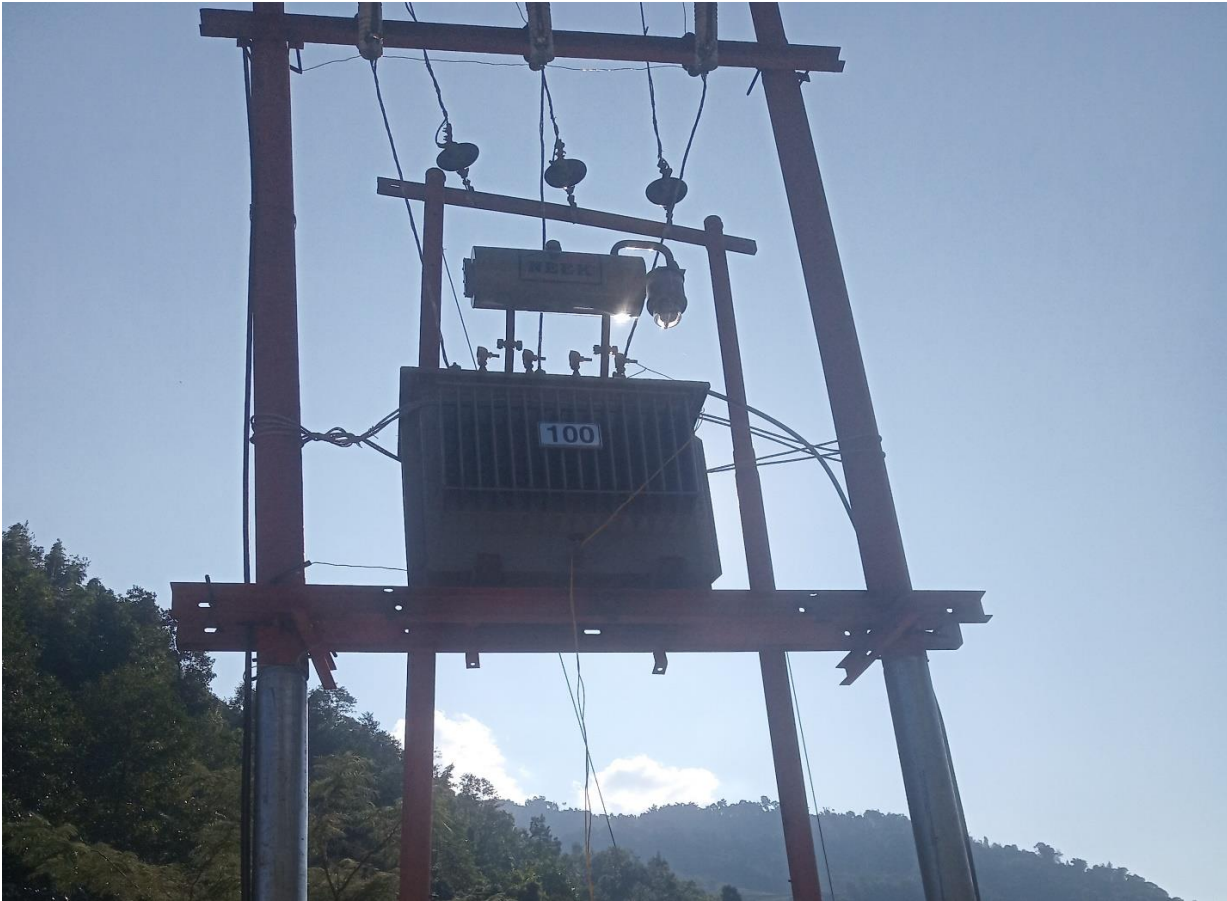
Figure 5: Transformer for construction power
